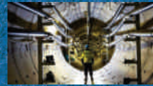
UNDERGROUND ELECTRIC SYSTEM
